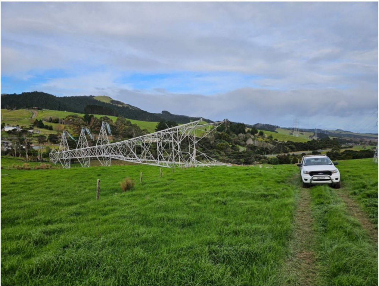
Figure 5: Collapsed tower 130 near Glorit
